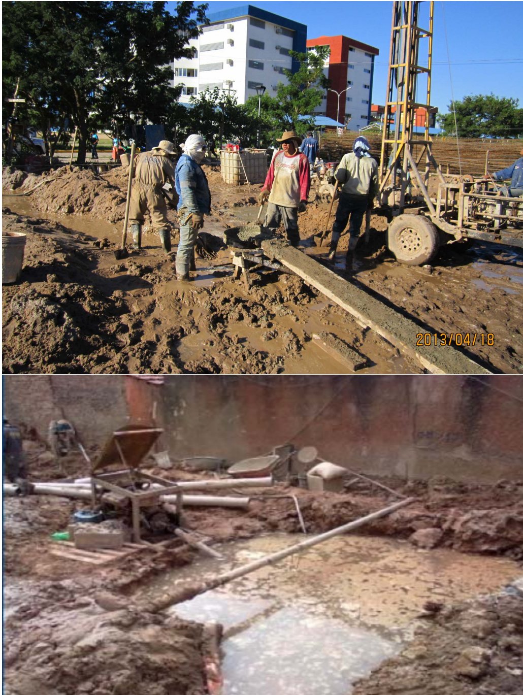
Fig. 2 Photos from a construction site in Santa Cruz, Bolivia, showing the rig and collection pit
